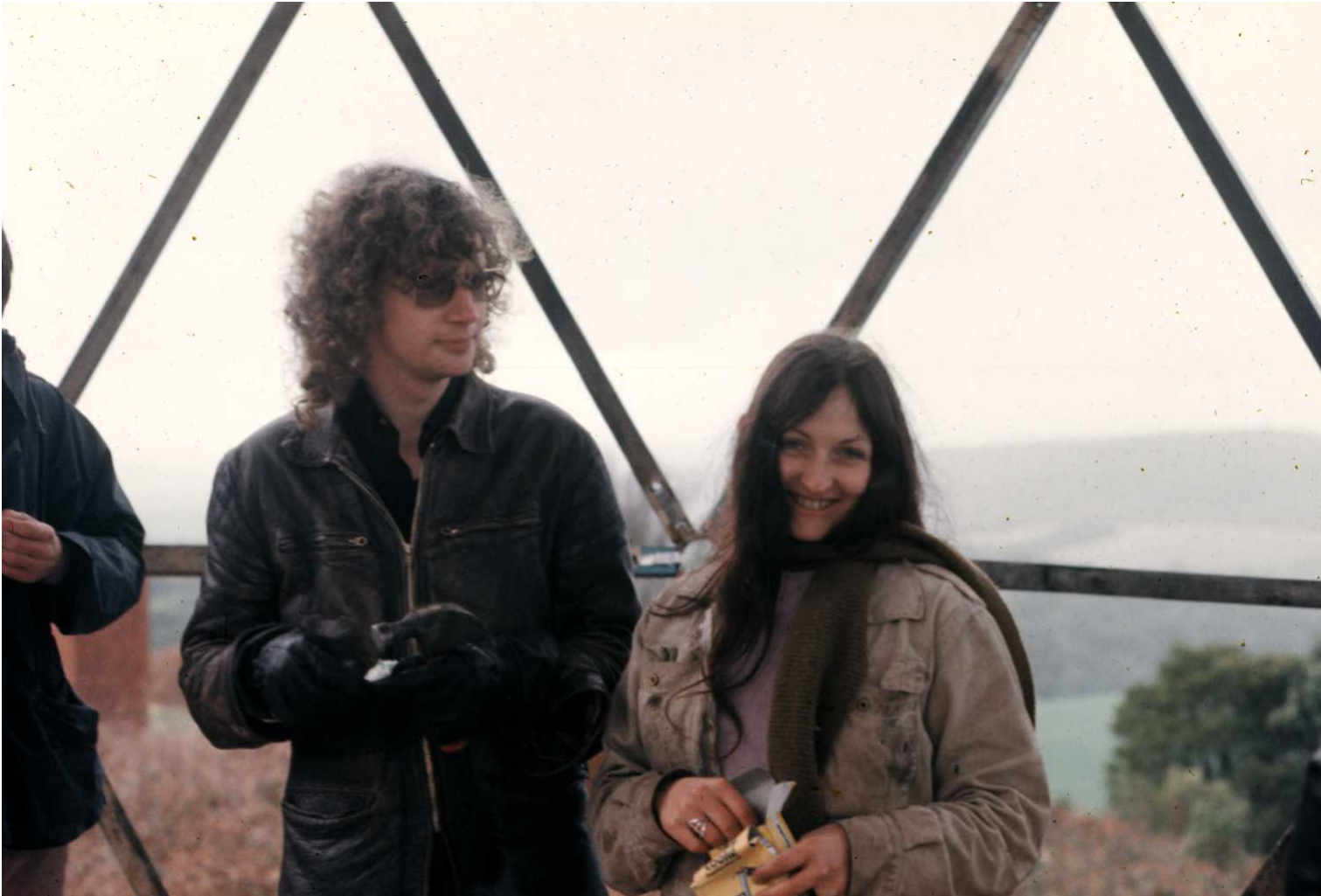
Lowen and Morgan. Building of the Domes at Beech Forrest in the Otway Ranges. Aug 1974
